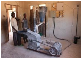
Electricity at the Mill
