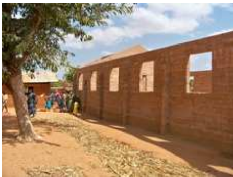
St. John's, waiting for a new roof
